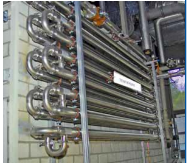
Mono-tubes mounted on a stainless steel frame
