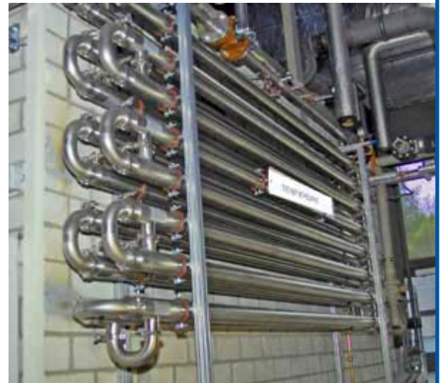
Mono-tubes mounted on a stainless steel frame
