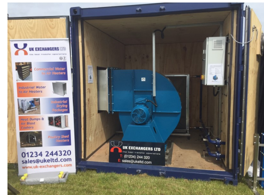
250 kW - G model in fully insulated container
